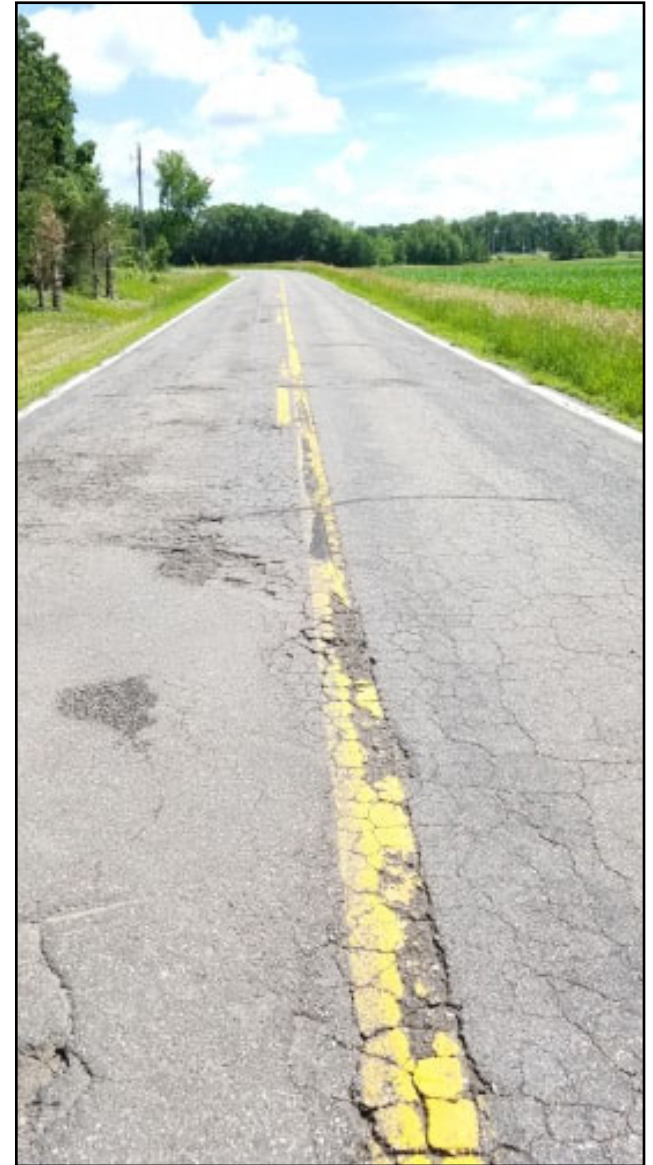
Photo of roadway pavement in poor condition. Photo courtesy of Saint Cloud APO.
