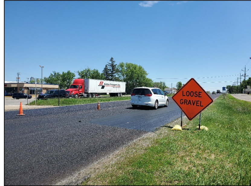
Figure 9: Photo vehicles traveling along CSAH 75 during road construction in Saint Joseph. Photo courtesy Saint Cloud APO.
