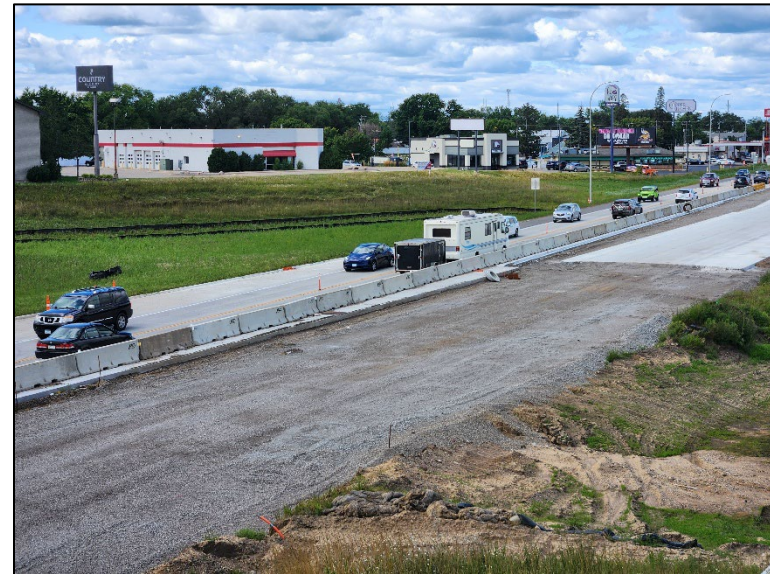
Figure 4: Construction on US 10 in Saint Cloud during the 2024 construction season. Photo courtesy Saint Cloud APO.
