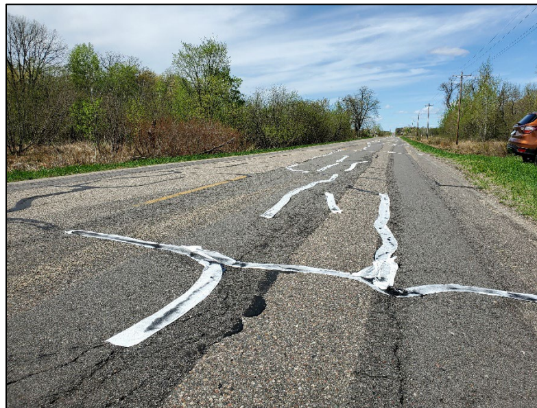
Figure 5: Photo of crack sealing work completed on Townline Road in May 2022. Photo courtesy Saint Cloud APO.
