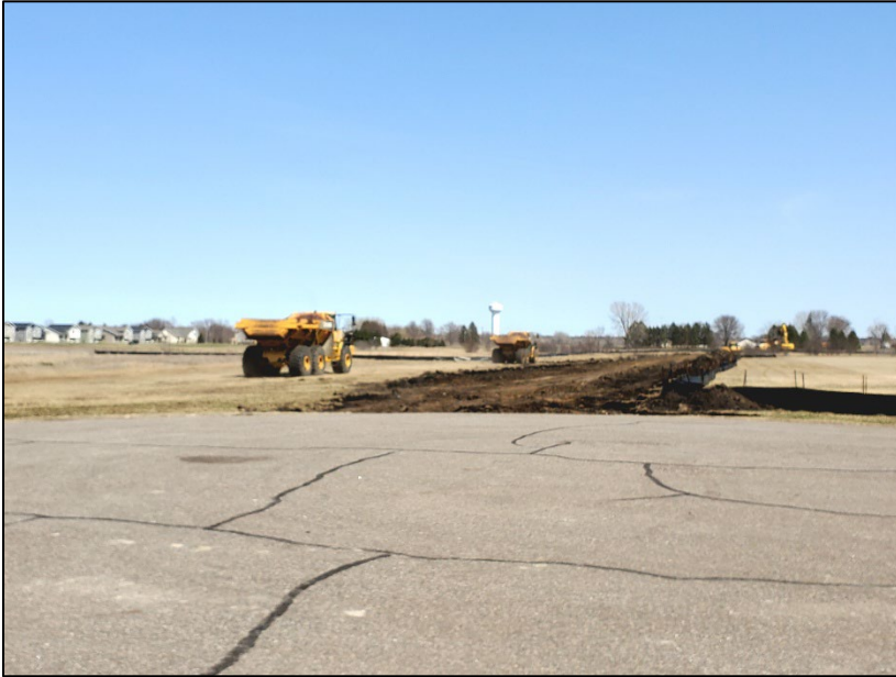
Figure 8: Photo of the construction of the Scout-Dehler Drive connection in Sartell. Photo courtesy Saint Cloud APO.
