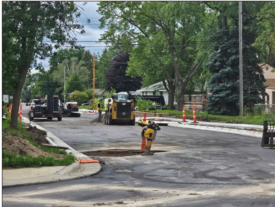
Construction crews completing work on 30 th Avenue in Saint Cloud during the 2024 construction season.
