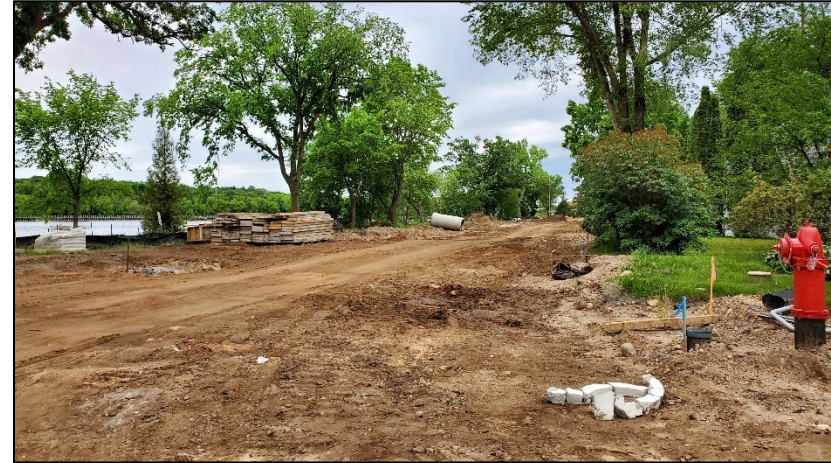
Figure 11: Photo of the 2022 roadway reconstruction project of Stearns CSAH 1/River Road in Sartell. Photo courtesy Saint Cloud APO.
