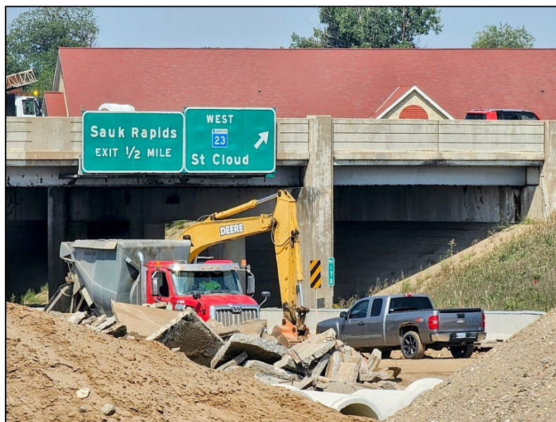
Figure 1.1: Crews working on the US 10/MN 23 interchange reconstruction project. Photo courtesy Saint Cloud APO.
