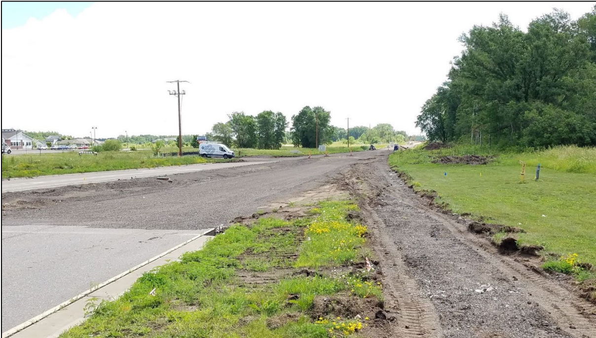
Figure 7.6: Construction of 33 rd Street S in Saint Cloud. Photo courtesy of Saint Cloud APO.
