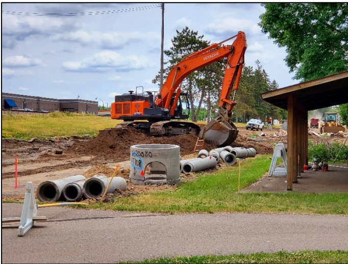
Crews working on reconstructing River Avenue N in Sauk Rapids. Photo courtesy of Saint Cloud APO.
