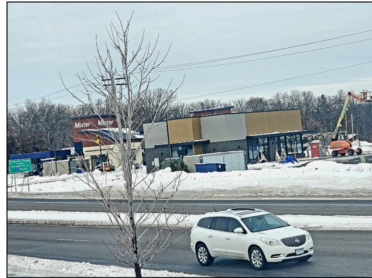
Commercial development under construction along MN 15 in Sartell. Photo courtesy of Saint Cloud APO.
