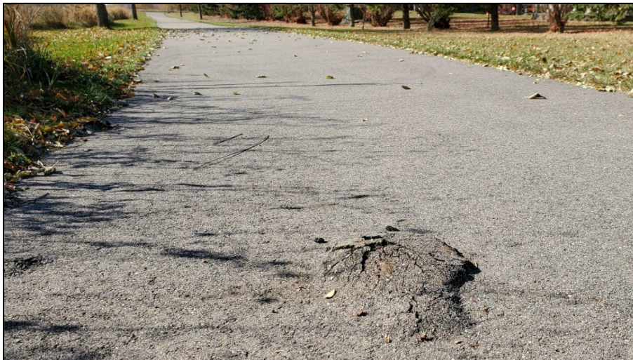
Figure 2.147 Pavement cracking on the Westwood Parkway Trail in Saint Cloud. Photo courtesy Saint Cloud APO.
