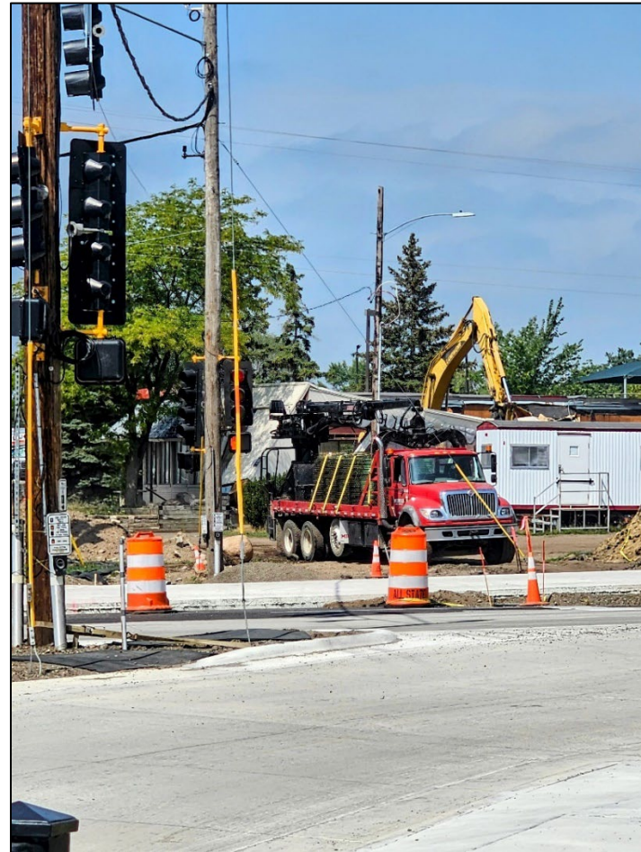
Figure I.5: Crews working on the reconstruction of the US 10/MN 23 interchange in Saint Cloud. Photo courtesy Saint Cloud APO.
