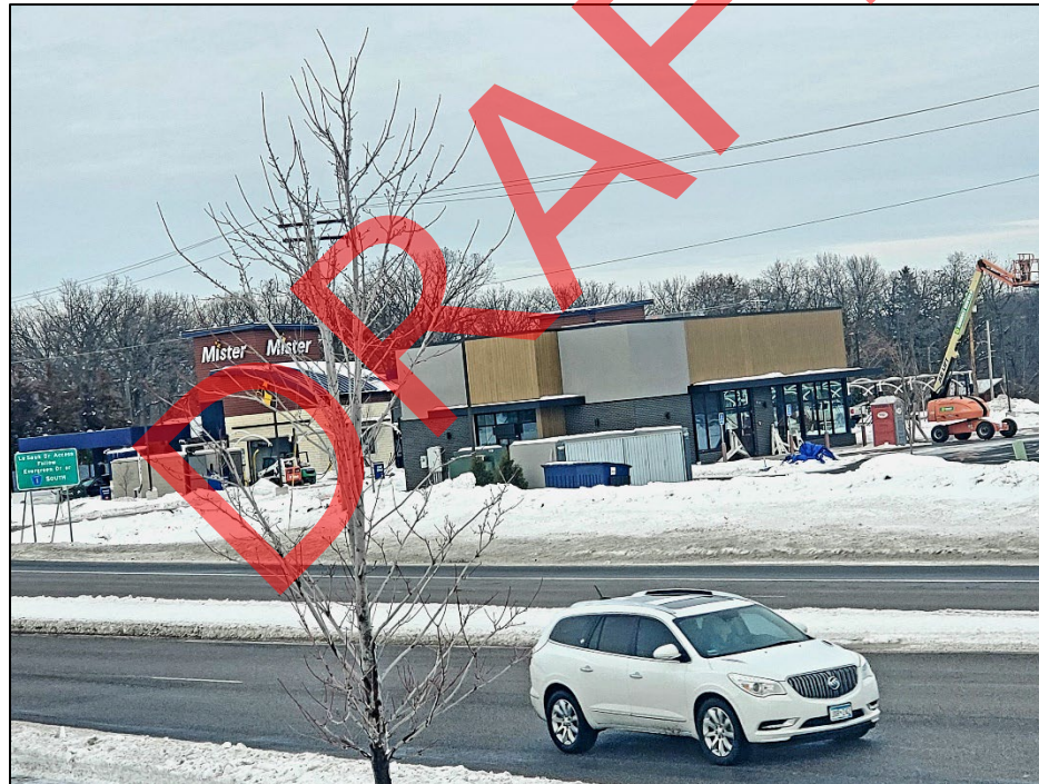
Figure 5.8: Construction of the new Chipotle along MN 15 near the intersection with Stearns CSAH 1 in the City of Sartell. Photo courtesy of Saint Cloud APO.
