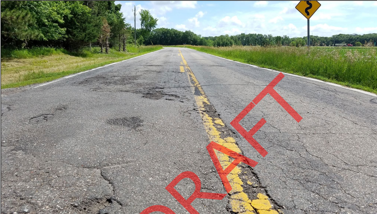
Figure 4.4: Cracking pavement along Graniteview Road in Waite Park taken in 2019. Photo courtesy Saint Cloud APO.
