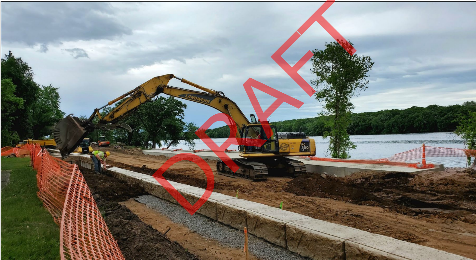
Figure 3.65: Example of reconstruction of Stearns County Road 1/Riverside Avenue N in Sartell. Photo courtesy of Saint Cloud APO.
