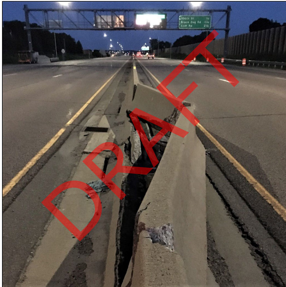
Figure 3.84: Concrete barrier buckling on Interstate 35. Photo courtesy of MnDOT.
