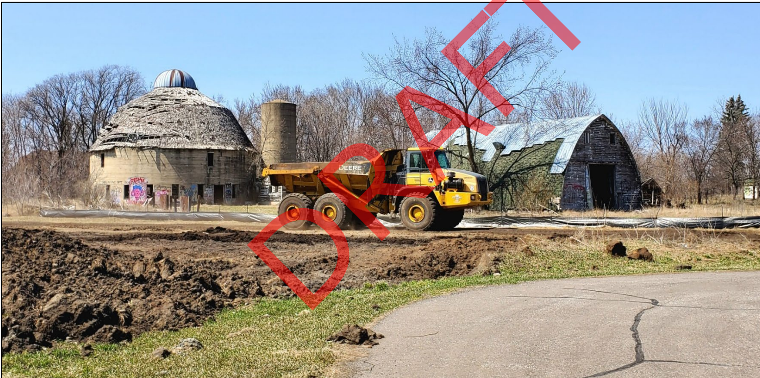
Figure 3.68: Construction of Scout Drive in Sartell. Photo courtesy of Saint Cloud APO.
