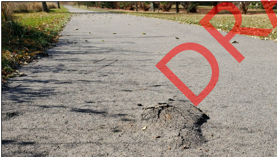
Figure 2.147 Pavement cracking on the Westwood Parkway Trail in Saint Cloud. Photo courtesy Saint Cloud APO.
