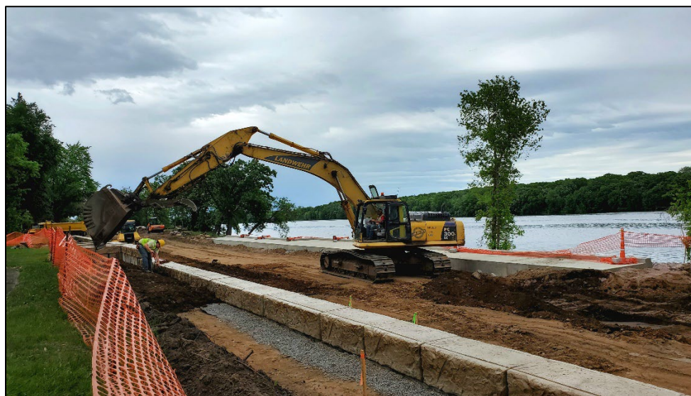
Figure 1.1: An excavator working on the 2022 reconstruction of Stearns County CSAH 1 in Sartell. Photo courtesy Saint Cloud APO.
