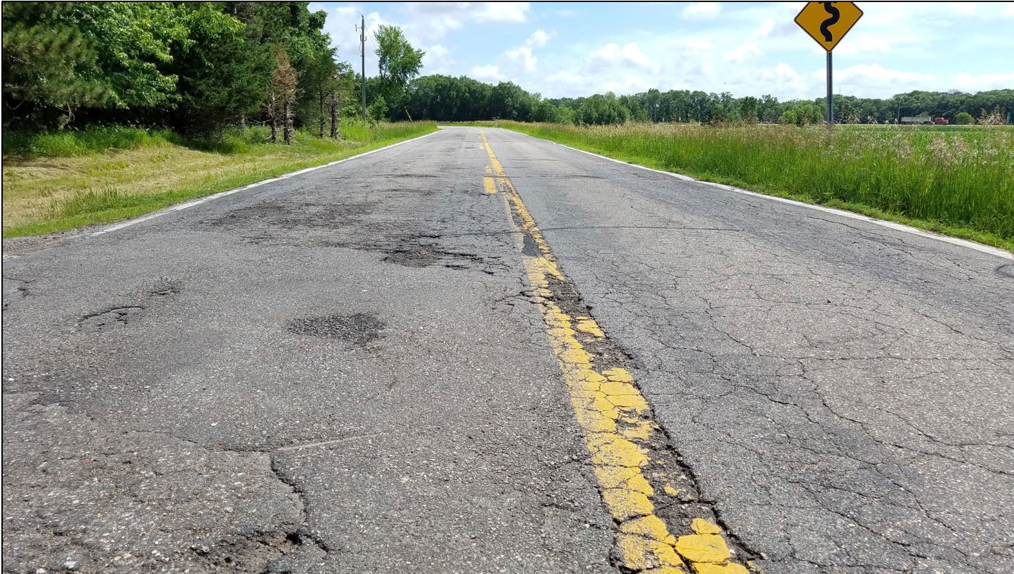
Figure X.4: Cracking pavement along Graniteview Road in Waite Park taken in 2019. Photo courtesy Saint Cloud APO.
