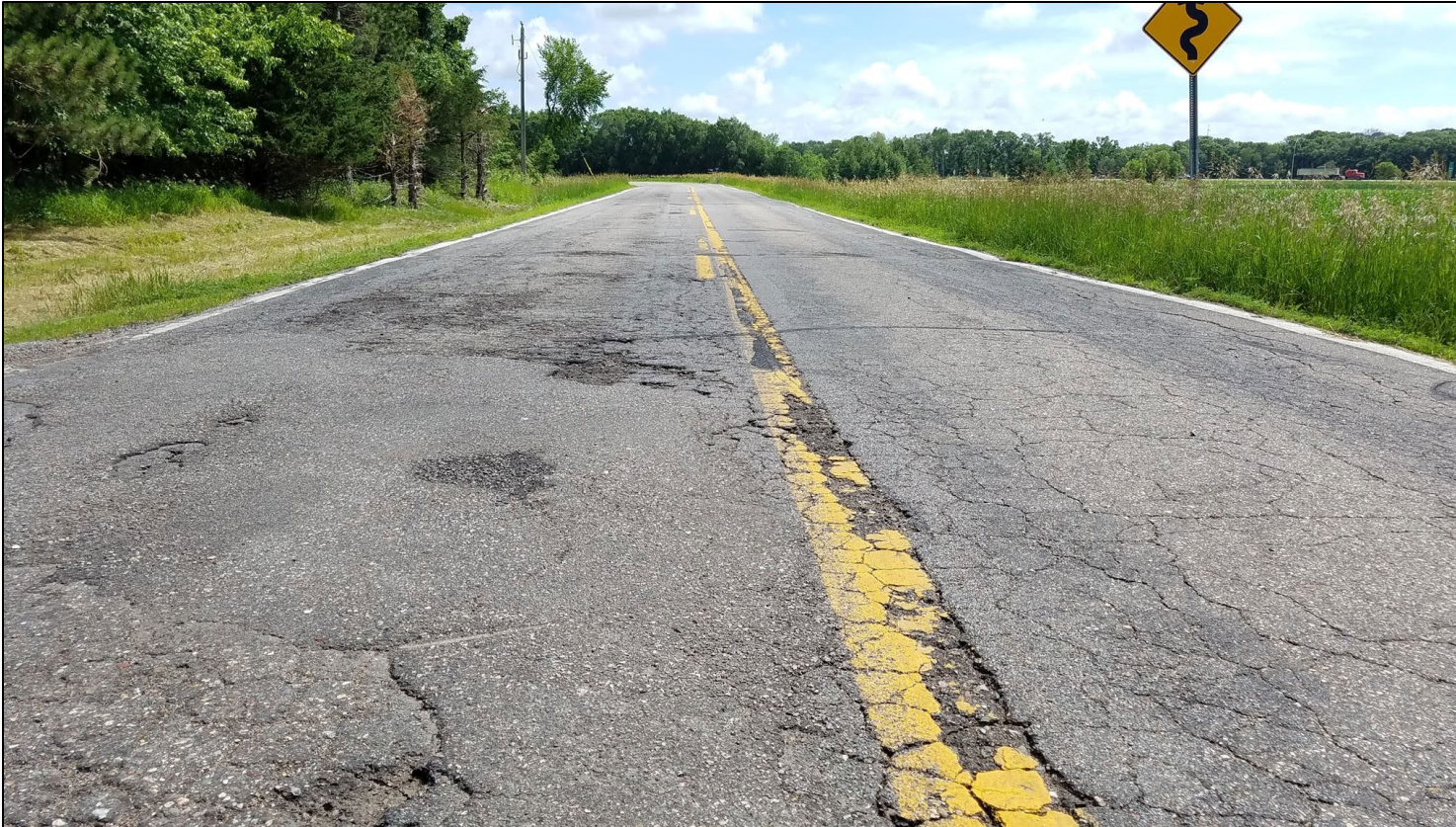
Figure X.4: Cracking pavement along Graniteview Road in Waite Park taken in 2019. Photo courtesy Saint Cloud APO.
