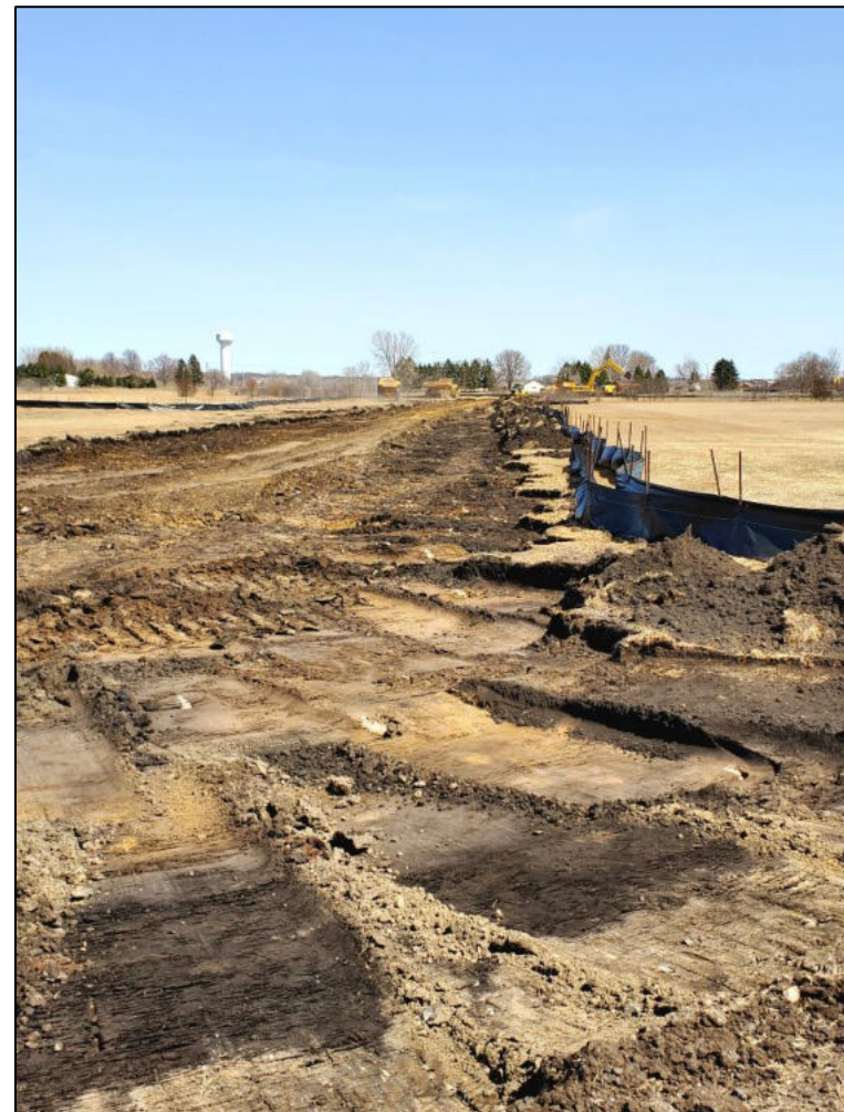
Figure I.5: Scout Drive to Connecticut Avenue S expansionary project construction. Photo courtesy Saint Cloud APO.
