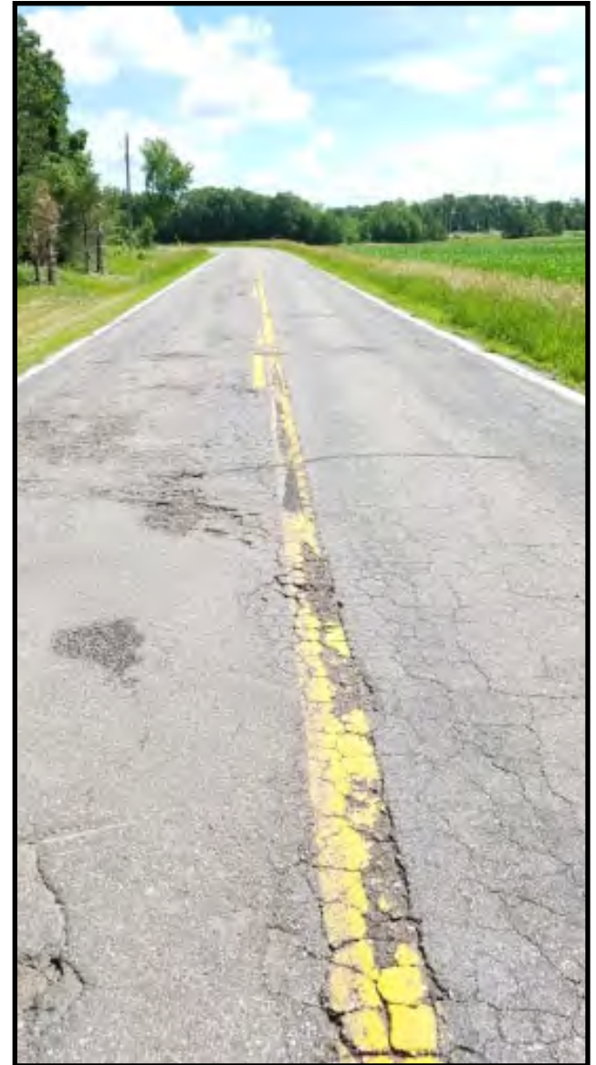
Photo of roadway pavement in poor condition. Photo courtesy of Saint Cloud APO.
