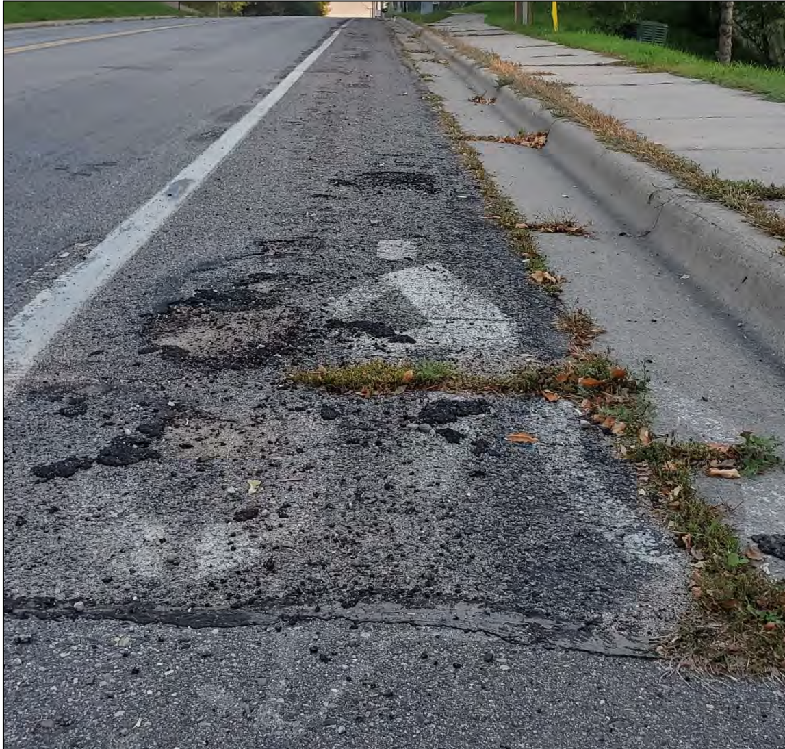
FIGURE 5.3 – EXAMPLE OF BIKE LANE IN POOR CONDITION IN SAINT CLOUD
